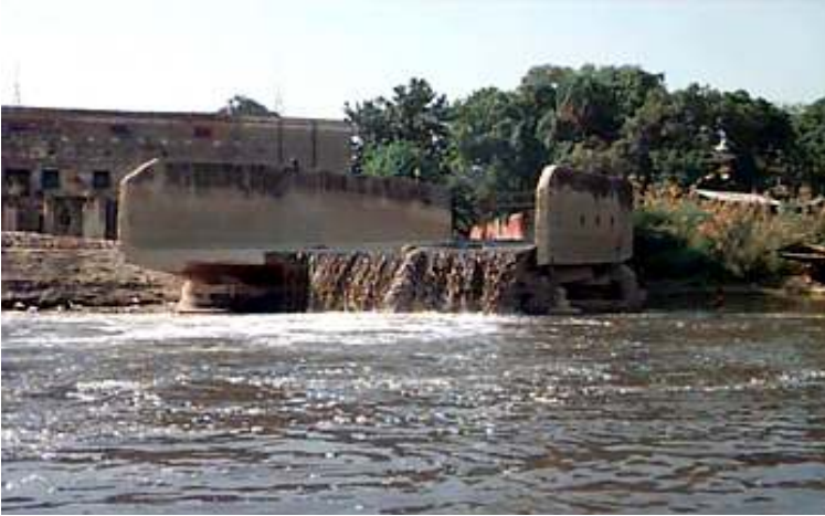
Sisamau drain discharging roughly 150 MLD of raw sewage into Ganga. This drain was not tapped under GAP I, is proposed to be tapped under GAP II.
