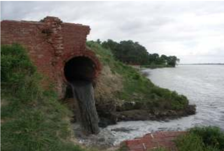
Dapka drain discharging raw sewage into Ganga. This is a failure of GAP I. Instead of reaching the treatment plant, the raw sewage is finding its way to river Ganga. Perhaps the trunk sewer is broken and clogged.
